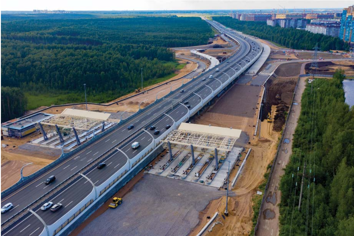
Transport interchange of the Western High-Speed Diameter (WHSD) highway at the intersection with Shuvalovskiy Prospekt. St. Petersburg
